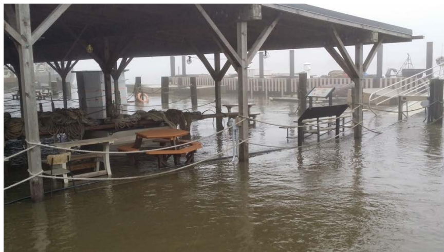
The fixed docks along the Delaware Bayshore and its tributaries, once perched above monthly high tides, are now flooded at full and new moons and during blow-in tides.
